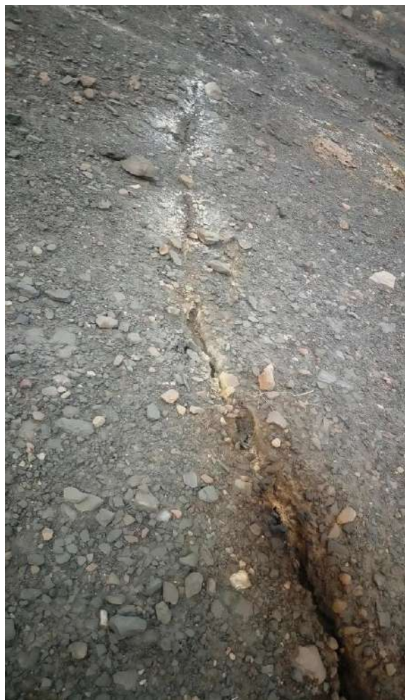
Figure 20: Fume cracks in the Bhulanbarari area.
